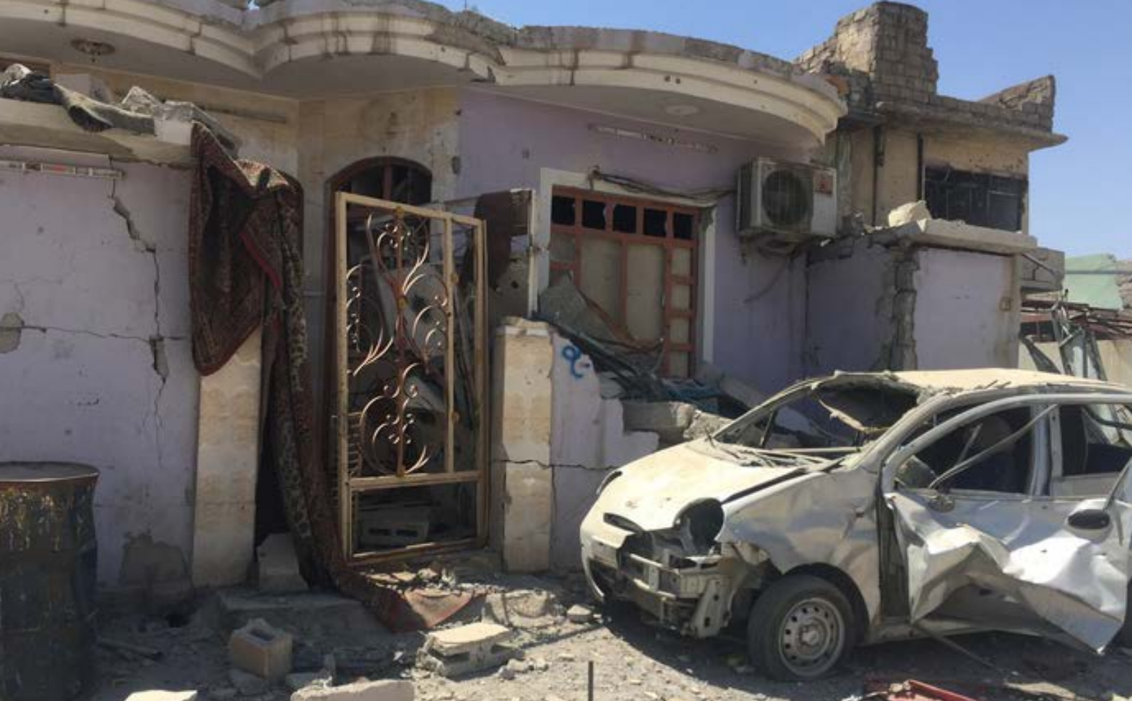
A damaged house in west Mosul following the fighting between the ISF and ISIS.. CIVIC/Sahr Muhammedally/June 2017.
